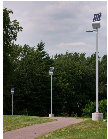
Carmanah EverGEN 1710 solar LED lighting illuminating the pathway at Thut Park in Madison, Wisconsin.
